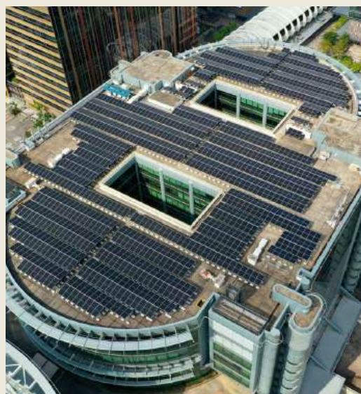
Photo credit: Sembcorp Industries
